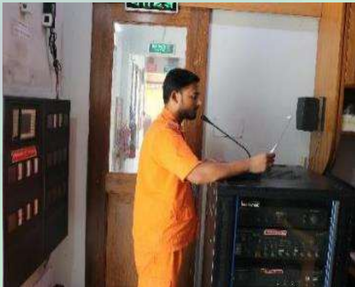
CENTRAL FIRE CONTROL & PA SYSTEM
