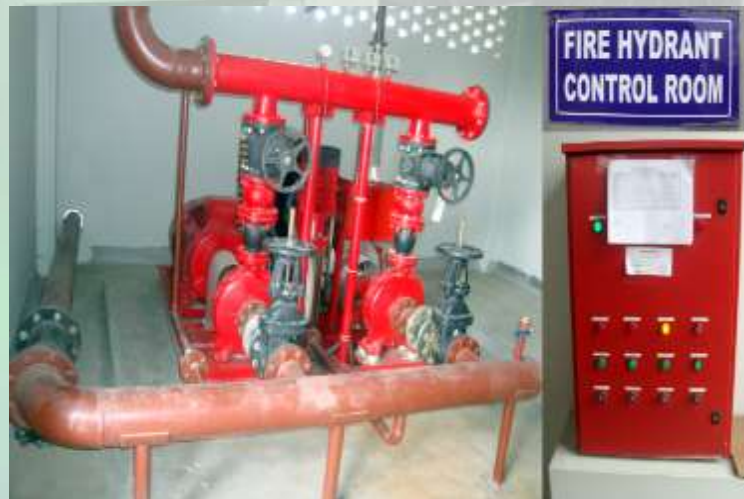
FIRE HYDRANT CONTROL ROOM
